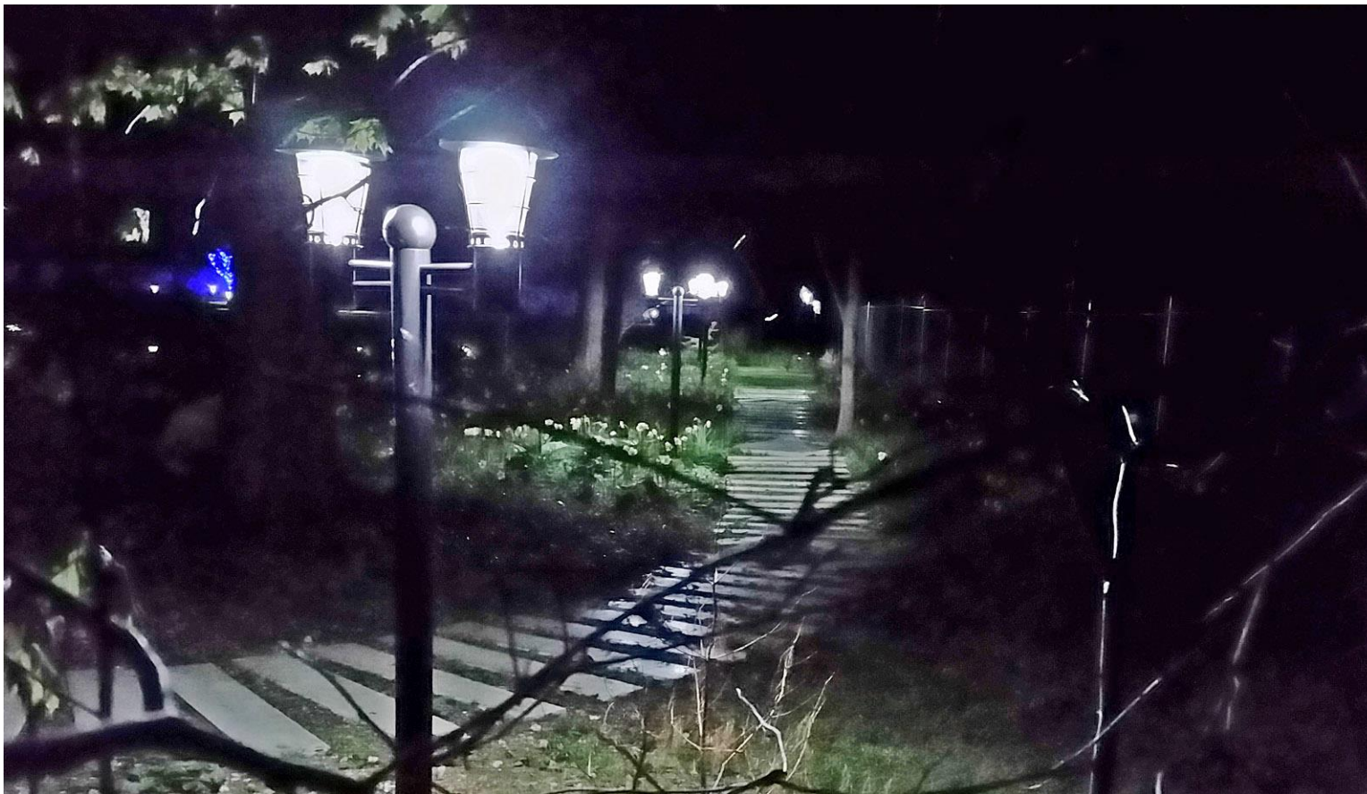
Lights are approx. seven feet high. Walkway follows protected stream at South property line.
